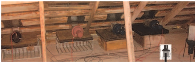
Figure 1. NaI(Tl) spectrometers installed beneath the tilt roof of the SKL experimental hall at Aragats station
